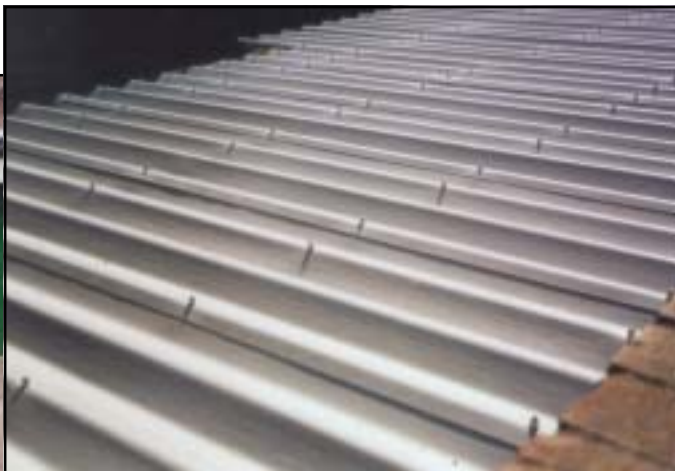
Refurbishment of garage block with FILON "DR" Doublesix by Caretec Building Preservations
