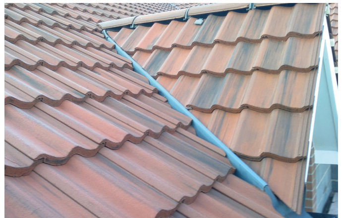
F. The completed installation: neat, tidy and effective – with minimal on-site time.
