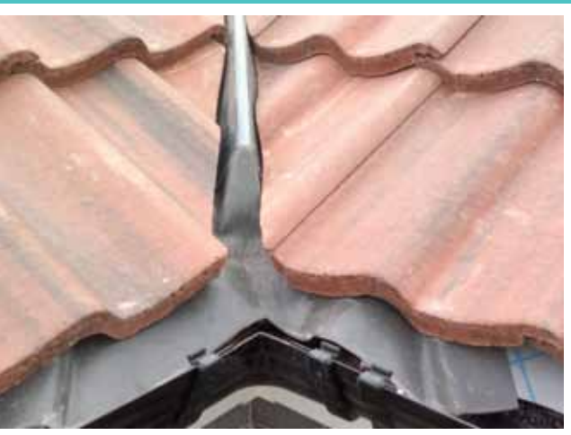
The eaves closure piece is cut to allow water discharge into the gutter.
