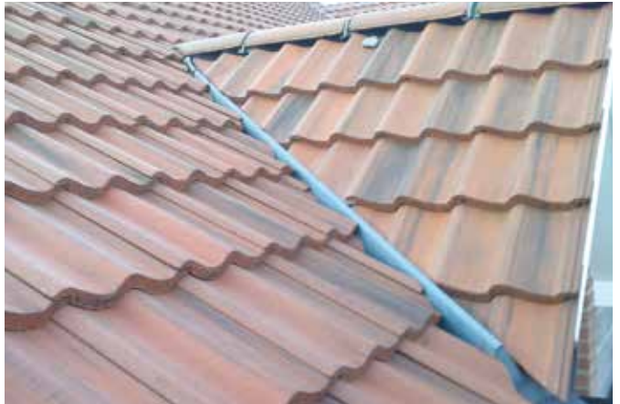
F. The completed installation: neat, tidy and effective – with minimal on-site time.
